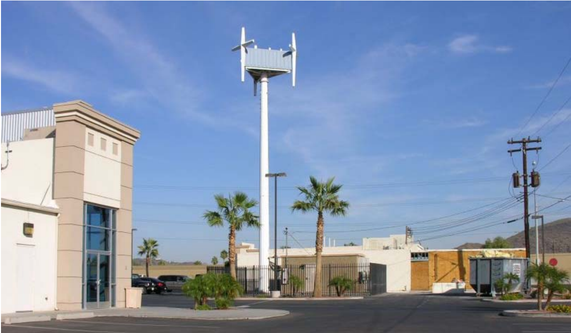
Figure 5: Semi-camouflaged Monopole wireless site in Phoenix, Arizona.
