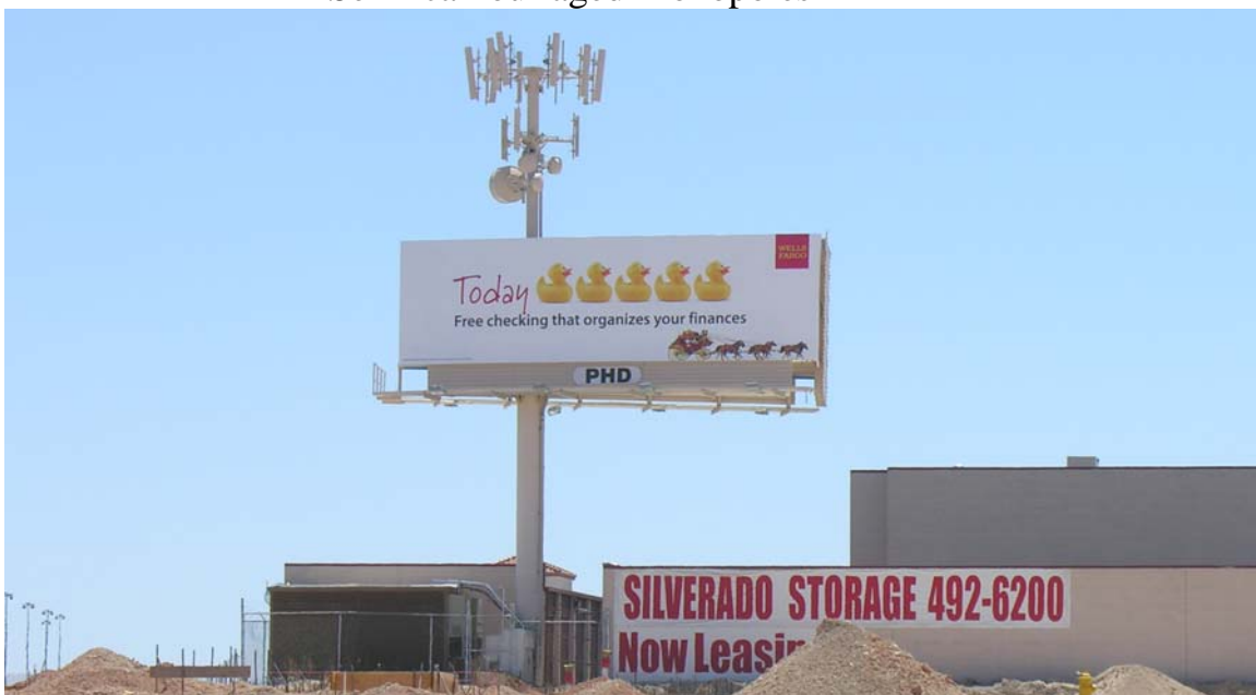
Figure 4: Semi-camouflaged Monopole/advertising billboard wireless site in Henderson, Arizona.
