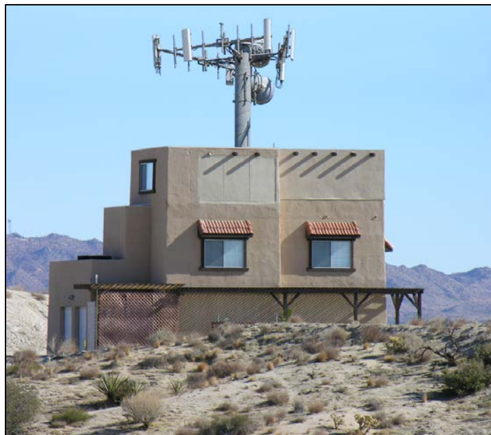
FIGURE 5: Photo simulation that shows a permitted modification under the PCIA formulation. The original site completely concealed all the equipment within the faux-house, whereas the hypothetical collocation does not “remove” the camouflage. (Source: Telecom Law Firm, P.C.)
